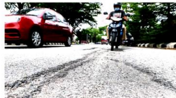
Publicly owned federal and state roads in a condition that is a bane for motorists. (left) in Klang, (right) in Klang.
