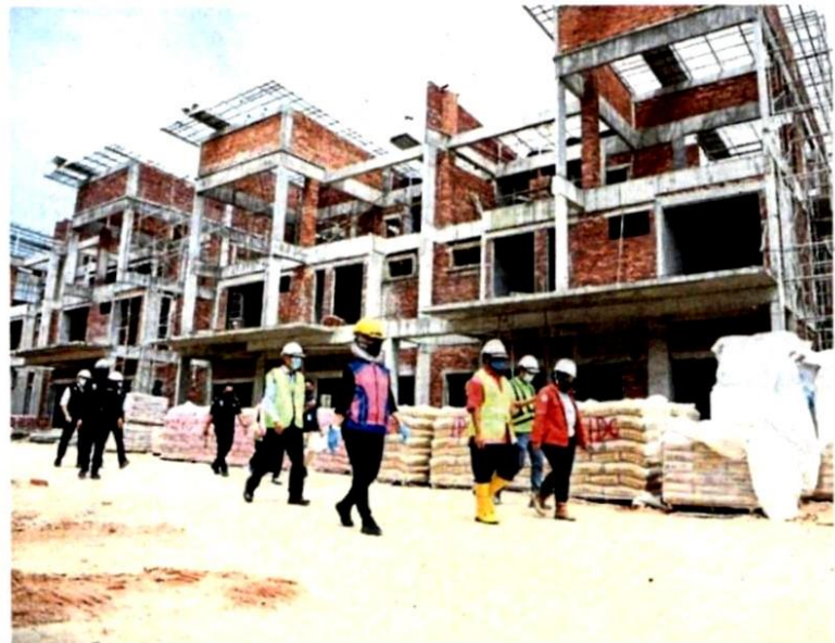
Worksites in Ampang being inspected during the joint operation headed by MPAJ.
